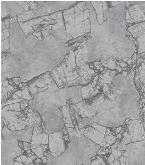
CONCRETO 90 ↔ ca. 99 X ↕ ca. 217 CM
